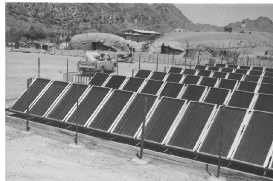
Fig. (10): Front view of solar collector assembly
